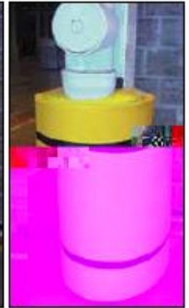
Protected with Concrete Wrap
